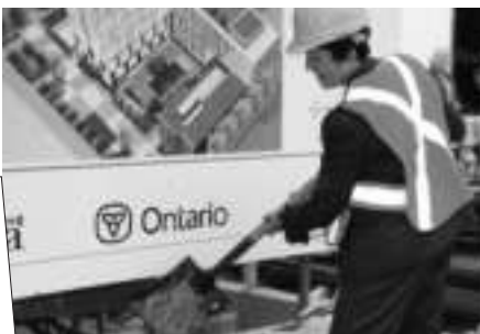
- Joan White, YWCA's Director of Housing Development pouring the cement into the foundation of the YWCA Elm Centre.
